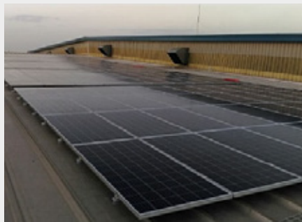
Solar power – 1,000 kw (IYM-CHE, India)
